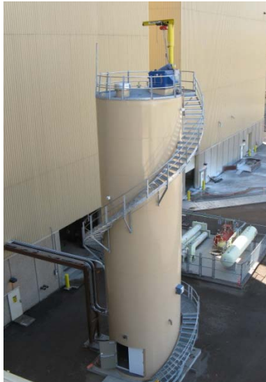
Activated Carbon Silo
